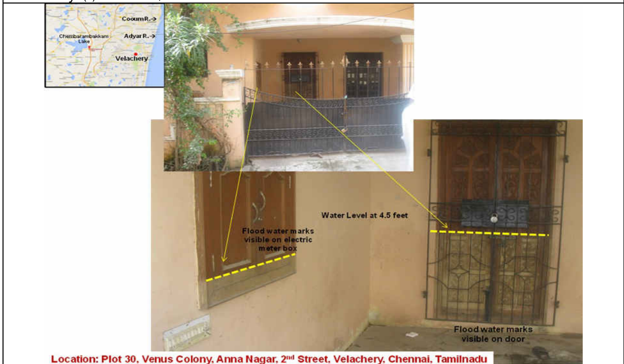
Fig-18 Flood water mark observed in doors, windows and electric metre box due to discolouration in one of the houses at Plot 30, Venus Colony, Anna Nagar, 2nd Street, Velachery. (c) NRSC/ISRO, 2015
