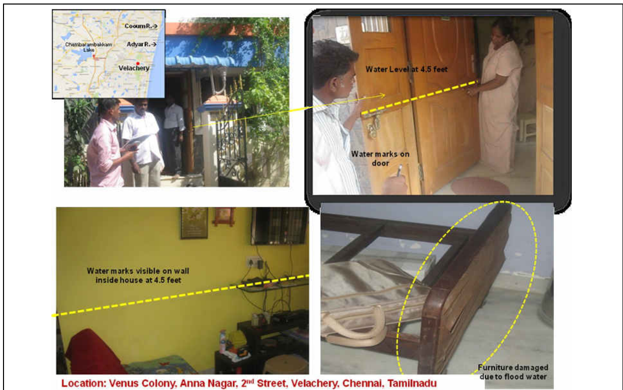
Fig-19 Flood water mark observed in doors, inside house and damage to furniture in one of the houses in Venus Colony, Anna Nagar, 2nd Street, Velachery. (c) NRSC/ISRO, 2015
